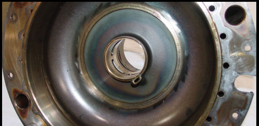
No. 5 bearing rear sump cover. Negligible deposits inside. Some light varnish deposits on flange indicating typical oil leakage from gaskets. Soot deposits from leakage on outside.
