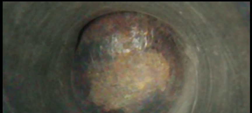
Oil supply tube. Negligible deposits. No reduction in area inside.
